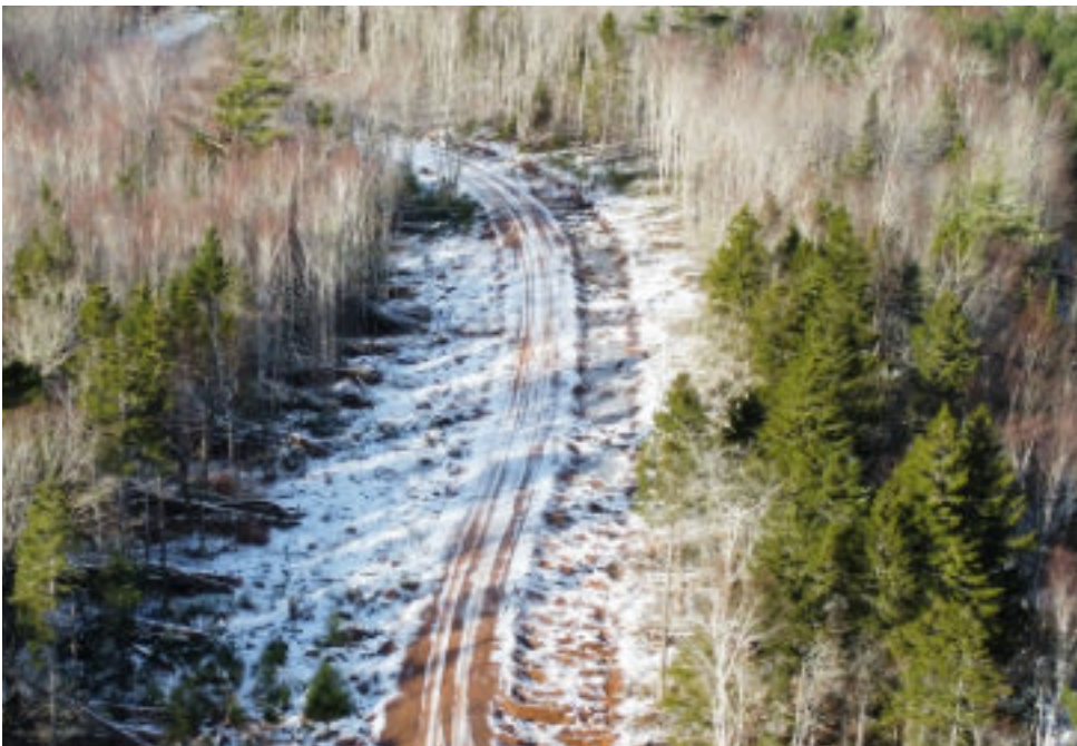
Drone image of the new road at Goldsmith Lake, 2022. PHOTO: NINA NEWINGTON.
